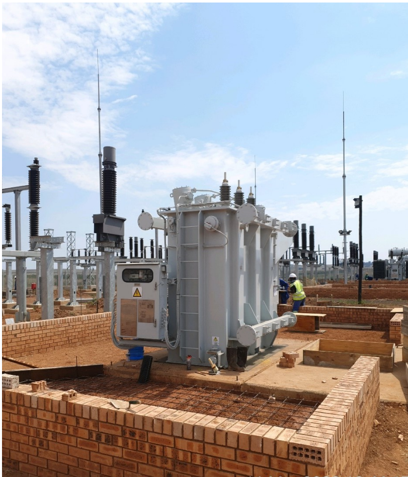
Figure 13: Example of Transformer installation with bund wall
